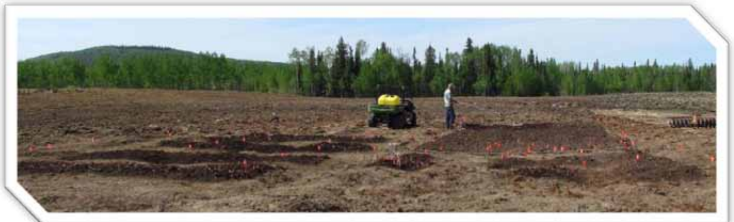
Installing the irrigation system became a priority when drought hit the field.
